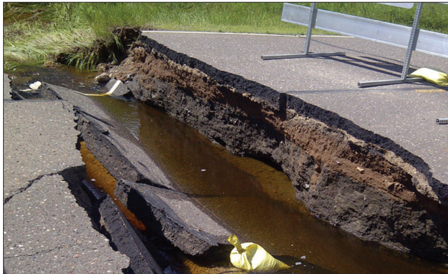
An entire section of County Road 13 near the Marathon Gas Station cracked and broke away, making it impassable.
